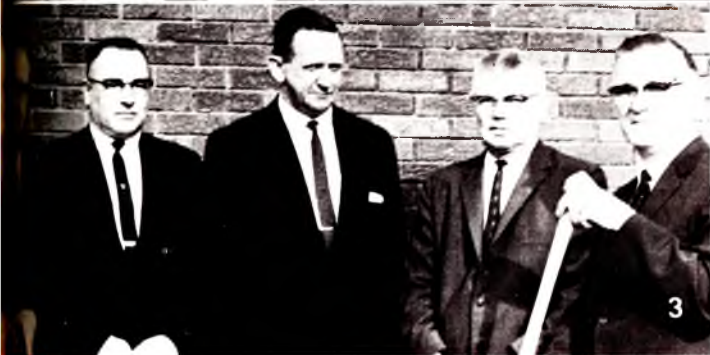
3 Sunday School Superintendent Willis Whitting (right) holds a shovel preparing to break ground for a new $33,000 annex for the Oil City, Pennsylvania, Church of the Nazarene. The two-story addition will provide a total of thirteen additional classrooms. Pictured, from left to right: Rev. Russell E. Lewis, pastor; Oscar Tarr, financial secretary and trustee; Harold J. Caldwell, trustee; Clyde Culbertson, board chairman and trustee; and Mr. Whitting.
