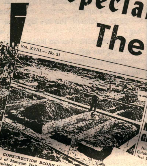
CONSTRUCTION BEGAN this week on the new east of Mangum Hall. The contractors hope to have the building completed by the opening of school next fall. The building will house 102 men.
